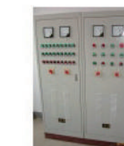
配电柜 POWER DISTRIBUTOR
